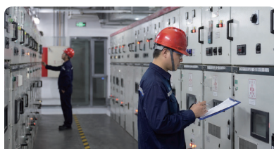
Electric Power & Utilities
